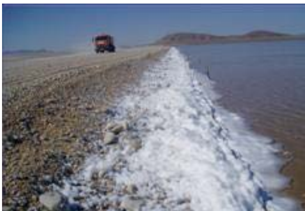
Figure 11: Risk of slope erosion
